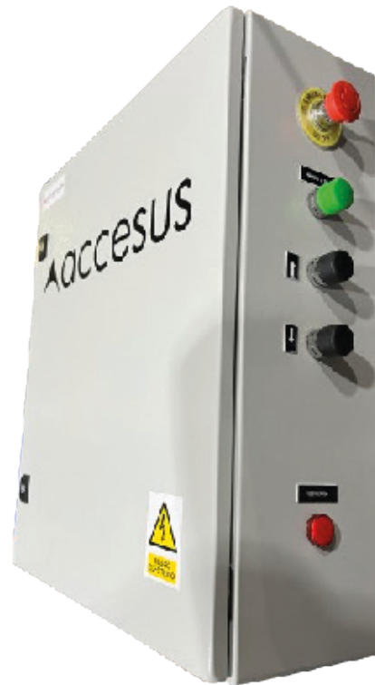
CONTROL PANEL FOR THE CONTROL OF 3 LEVA LIFTS
