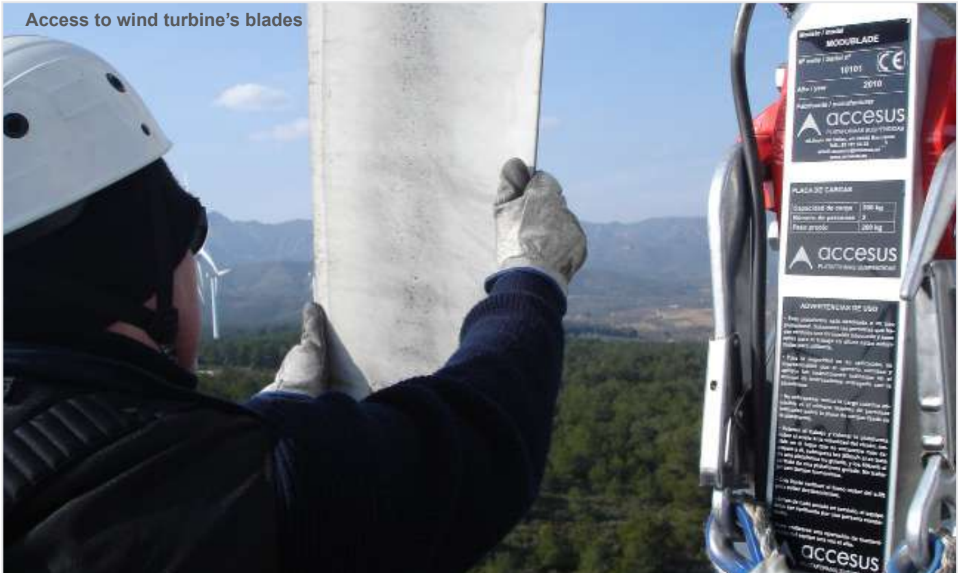
Access to wind turbine's blades
