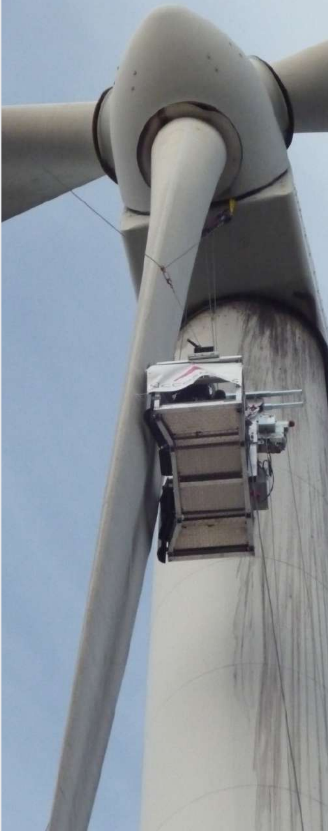
Access to wind turbine's blades
